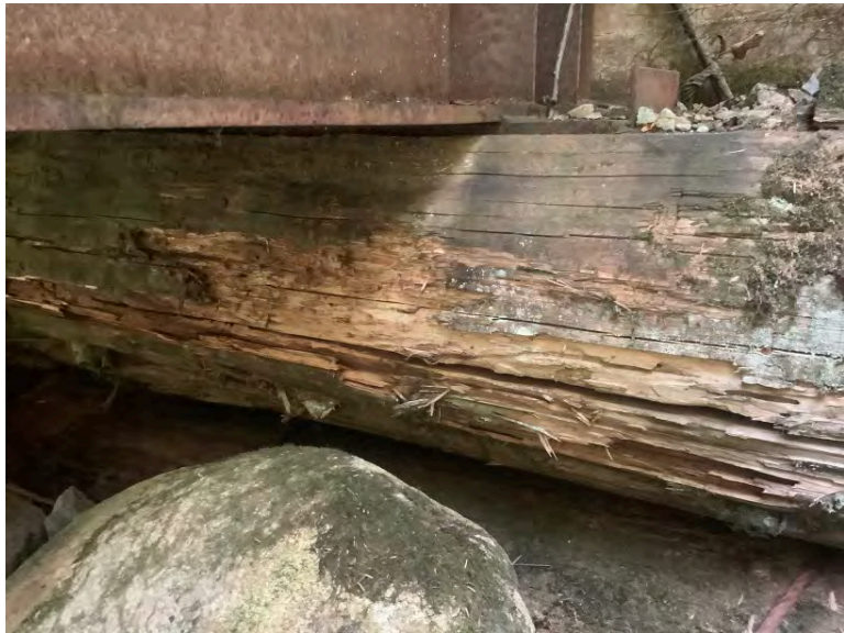
Upstream right bearing crack
